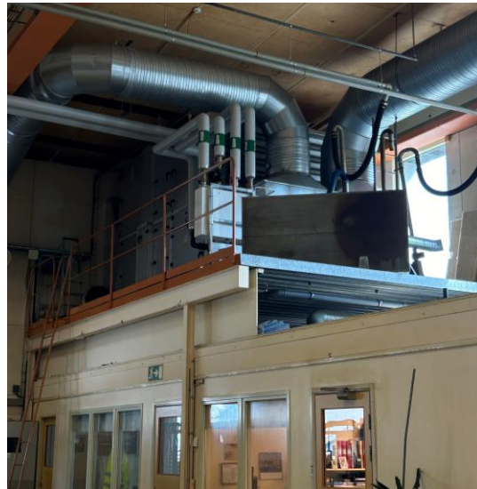
The ventilation system at the Hestra factory, Sweden
